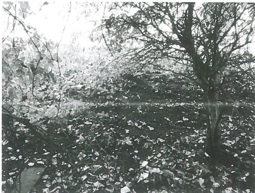
Plate 10. Loose soils at burrow on embankment to north of site Fox? Rabbit?
