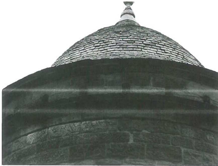
Plate 9. Dovecote showing crevices at wall head and gaps under slates
