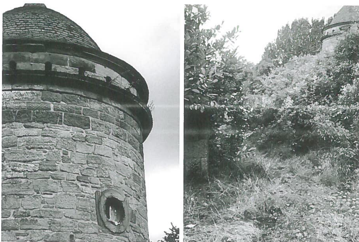
Dovecot in need of maintenance
